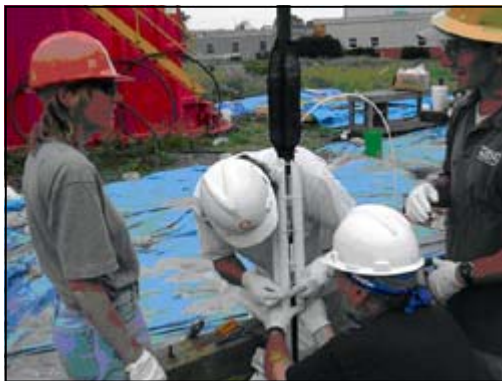
USGS scientists assembling a sampling device for insertion into a well to enable long-term sampling from fractured zones at the NAWC site in West Trenton, N.J.
